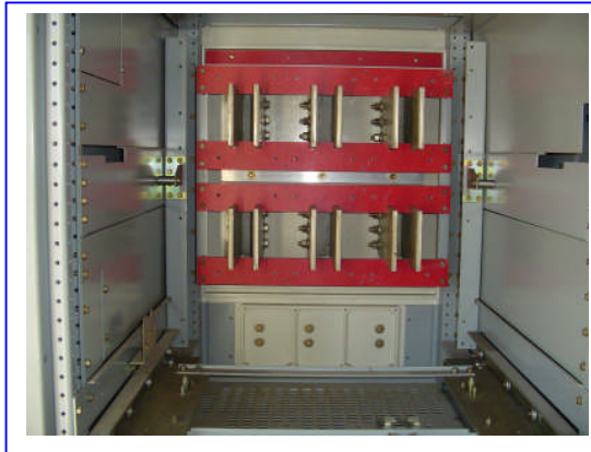
Fig. 6: The horizontal test setup was designed to simulate rear-fed equipment like this unit.
